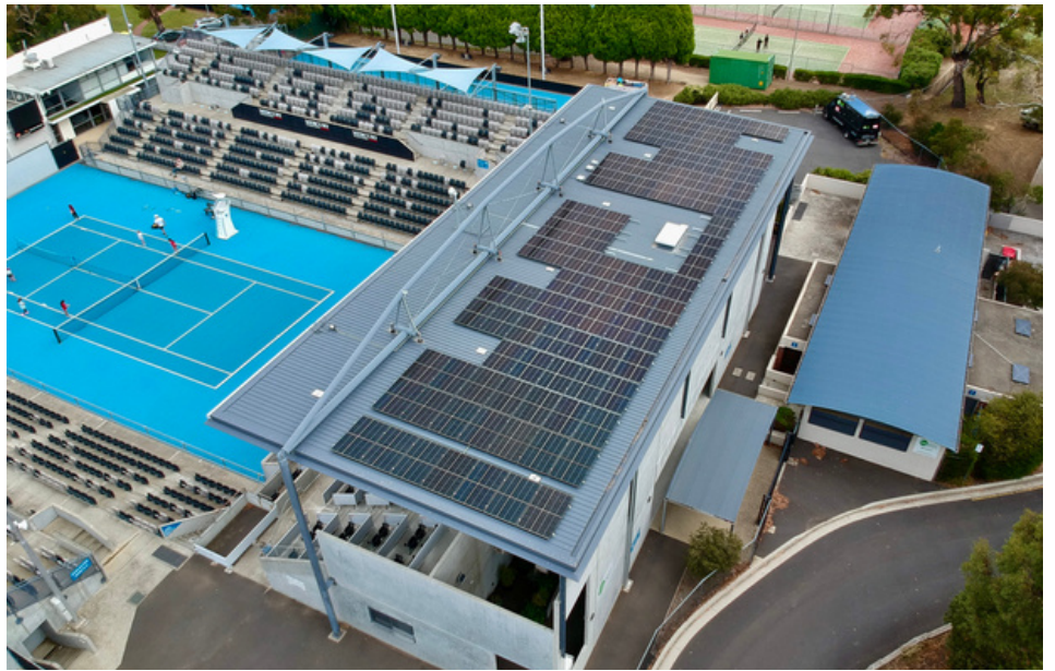
Solar system on the Northern Grandstand
